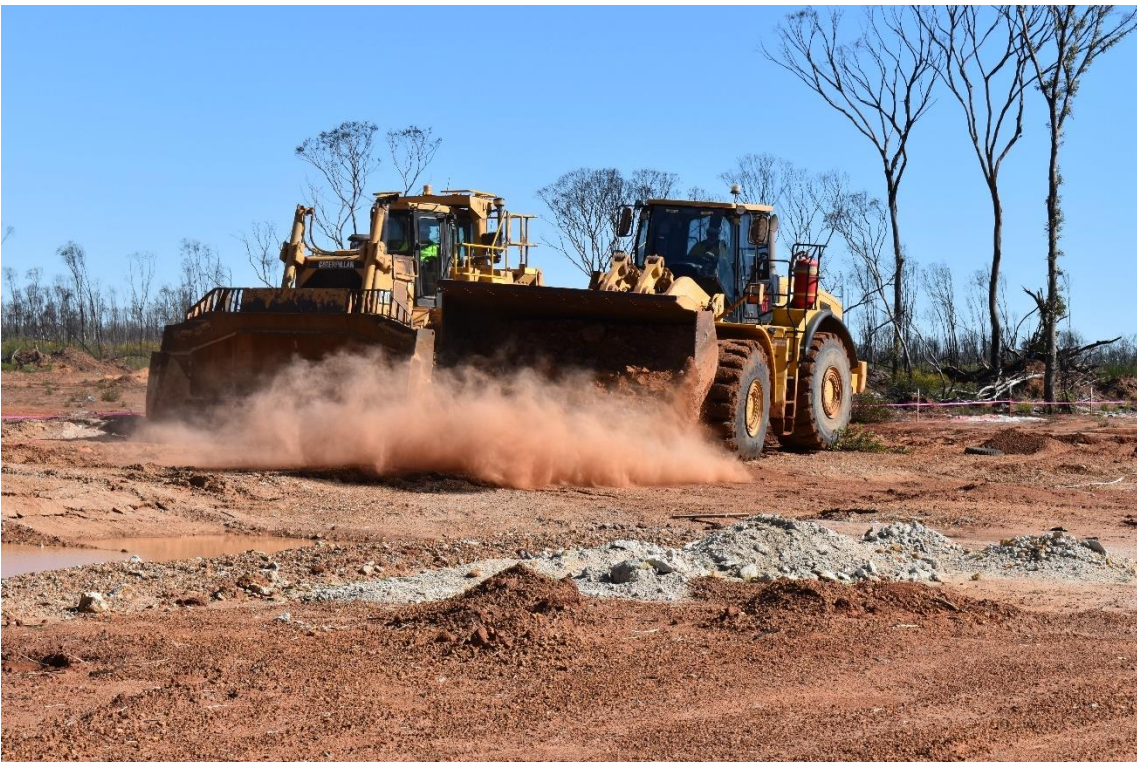
Figure 4: Dozer and Loader commence pushing back top soil at Bulk Sample Pit.
