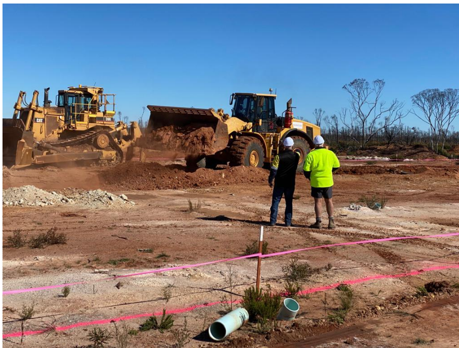
Figure 3: Dozer and Loader commence pushing back topsoil at Bulk Sample Pit, Kat Gap.
