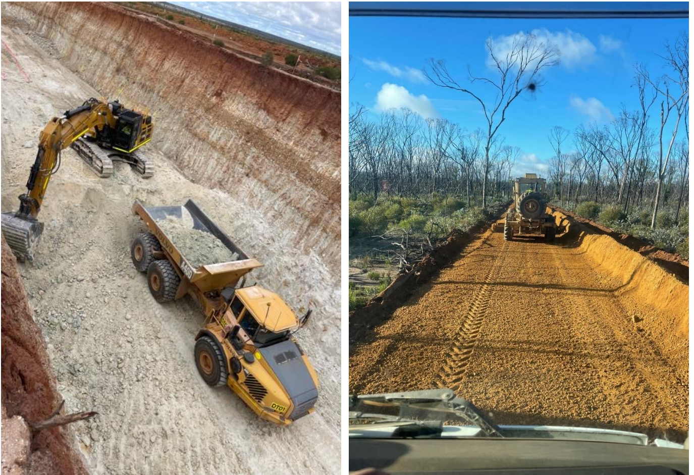
Figure 3: Excavator loading dump truck & construction of road to new mining camp site
