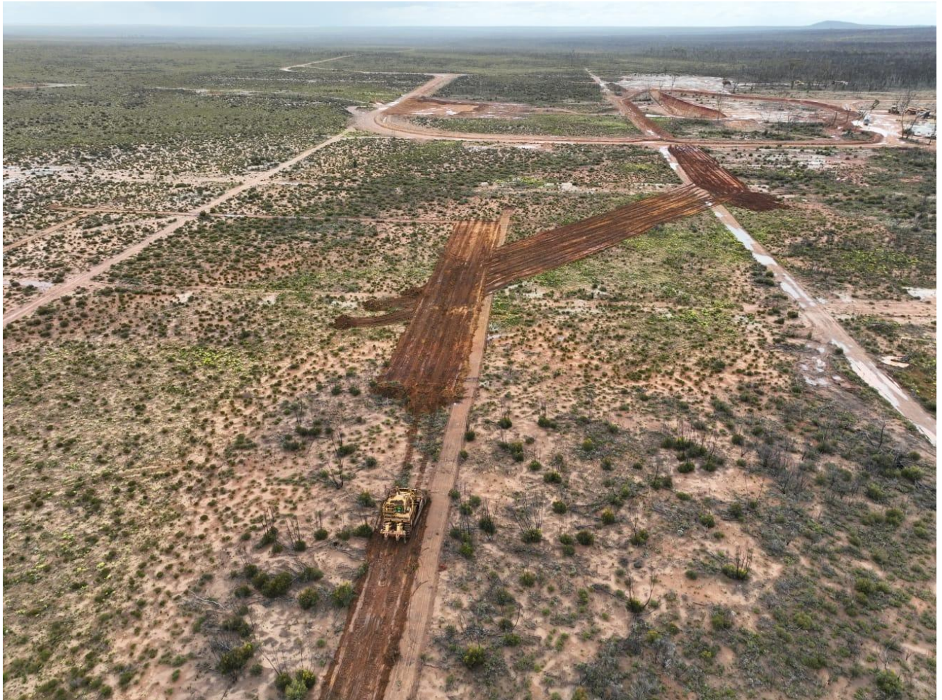
Figure 3 (below): Bulldozer clearing the ROM Pad and Haul Road at Kat Gap.
